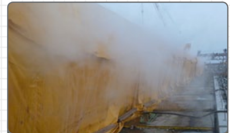
Traditional tarping method shown, which resulted in steam loss & rising fuel costs.
